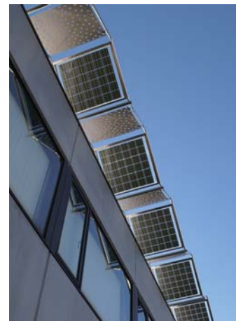
Canopy with PV system We arranged designed punching panels to the north.
